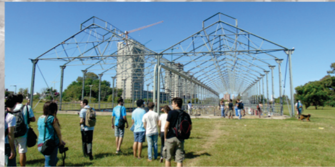
Parabolic solar collectors on the roof
